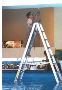
Monon: Using an electric tool, in a pool, with a metal ladder. David Monon: Standing barefoot on the ladder while using it.
